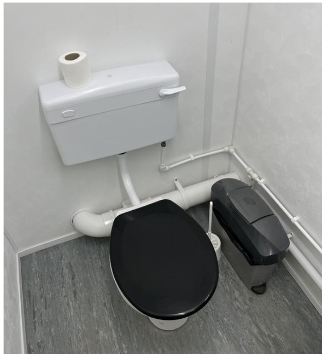
Sanitary bin & toilet brush
